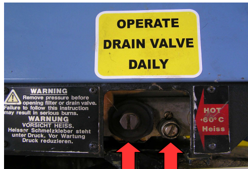
TANK FILTER DRAIN VALVE
